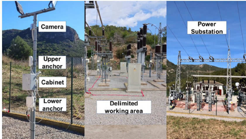
Figure 2: Left: monitoring field devices. Centre: physically delimited area. Right: outside view Ecogarraf substation
